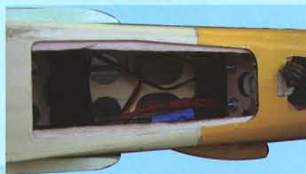
22A- Battery locations
