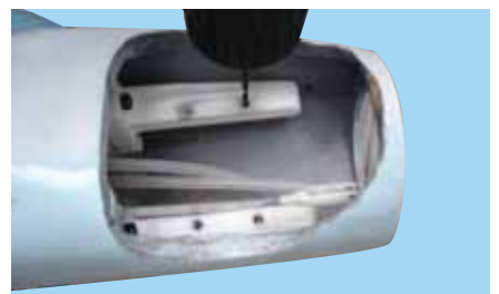
12D - Drill 3/32 in. (2 mm) pilot holes at right angles through the beams
